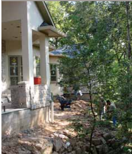
Prior to pouring the foundation of the house, the builder reinforced the ravine side of the property with machine-placed moss rock boulders.
